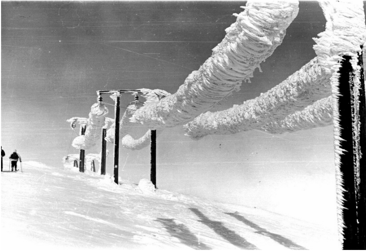
Fig. 1.1 Rime icing on a 22 kV electric power line in Norway April 1961, 1 400 m above sea level. The ice load was measured to 305 kg/m (Photo: O. Wist, reproduced by permission of S. M. Fikke)
