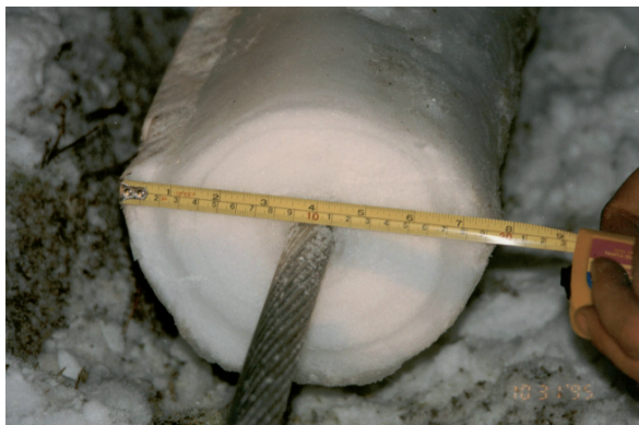
Fig. 1.2 Wet snow accretion on a collapsed power line in Iceland (Reproduced by permission of Á. Elíasson, Landsnet, Iceland)
